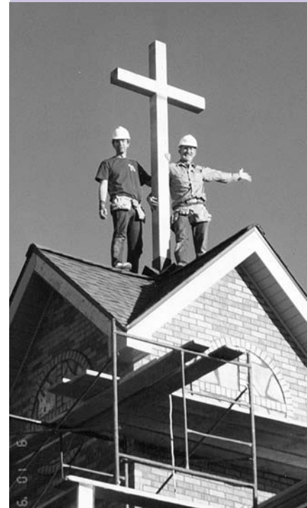
Howard, on right, obviously not awed by heights, stands tall on one of his early projects at Messiah Lutheran in Aurora, Nebraska.
