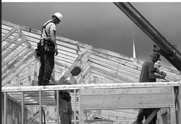
Howard McCartha, project manager during construction of the addition to Trinity Lutheran Church, Platte, South Dakota,
