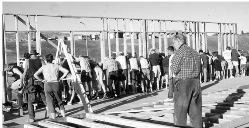
More than 70 members of Celebration Lutheran Church, East Wenatchee, Washington, worked with the Mission Builders on the first wall-raising for their facility.
