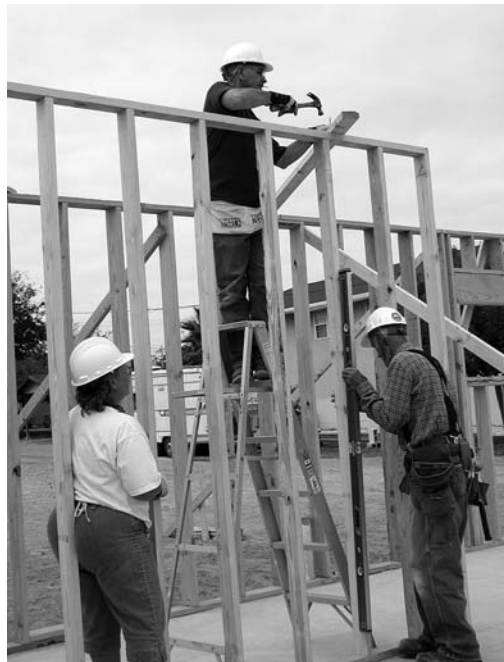
The Rev. Dr. Ray Tiemann, bishop of the Southwest Texas Synod (on the ladder), joins Patty Weber and Roy Doell, construction manager, at the Eagle Pass construction site.
